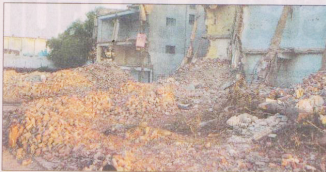
The south civic body will send trucks to lift debris once it receives a call on its helpline.
